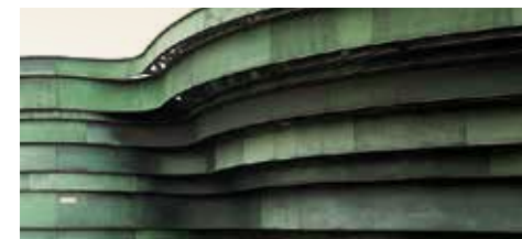
Jubilee Line Vent, photograph by Vera Dohrenbusch
